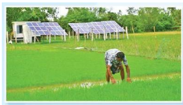
Figure 29: Solar Pump System in Rangpur District
