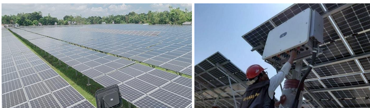
Figure 28: Bangladesh's Largest (73 MW) Solar Power Plant, Mymensingh
