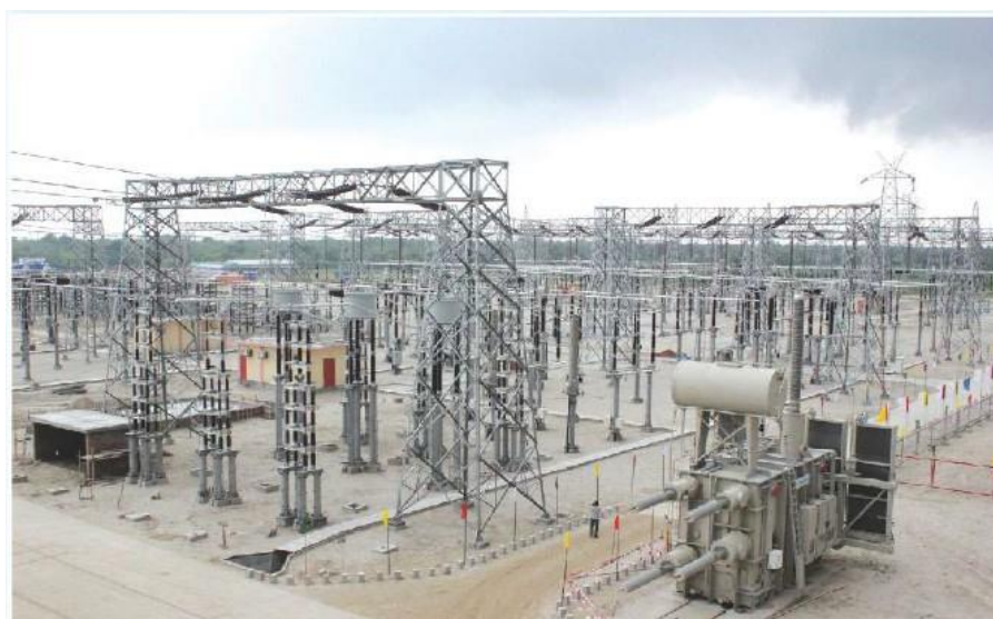
Figure 25: Bangladesh India Power Transmission Plant, Bheramara (Kustia)
